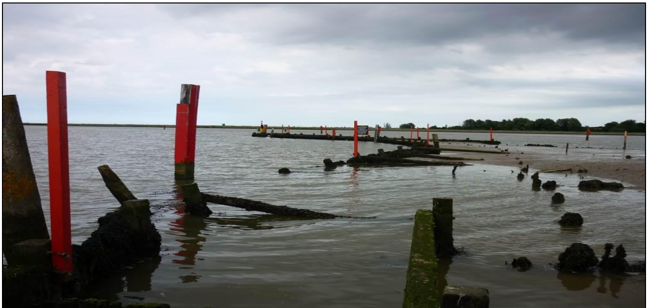
Photo: Failing jetty piling taken in August 2014
