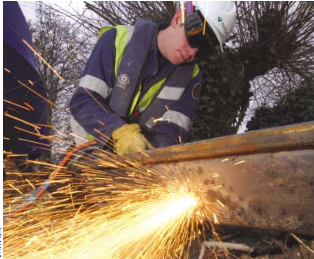
Let the sparks fly! Work on the new piling in the mooring basin at Upton Dyke, off the River Bure
