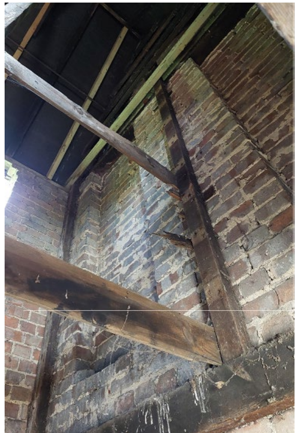
Evidence of smoke inside
