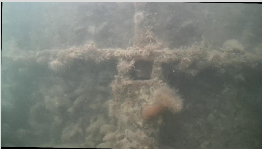
Marine growth on external lock gate penstock.
