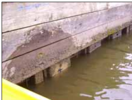
PHOTOGRAPH 1 SHOWING EXISTING STEEL SHEET PILES WITH TIMBER CAPPING TO BE RETAINED IN SHORT TERM (CHAINAGE 5330 - 5390m)
