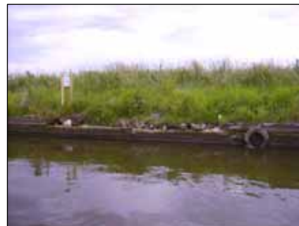
PHOTOGRAPH 2 SHOWING EXISTING DILAPIDATED STEEL SHEET PILES TO BE REMOVED (CHAINAGE 5390 - 5460m)
