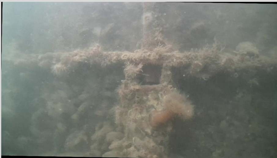
Marine growth on external lock gate penstock.
