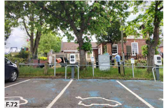
Figure 72: Photo of electric charging spaces at the Church Plain Car Park.
