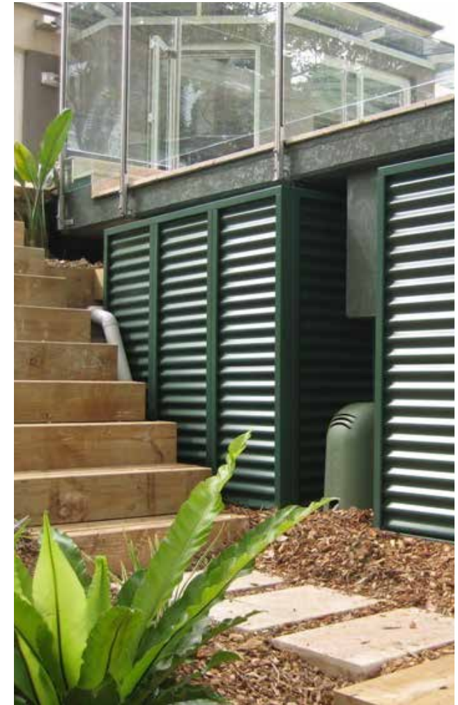
Figure 97: Example of a modular water tank
