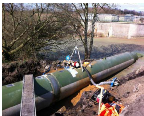
Figure 3: River Wissey fish pass siphon
